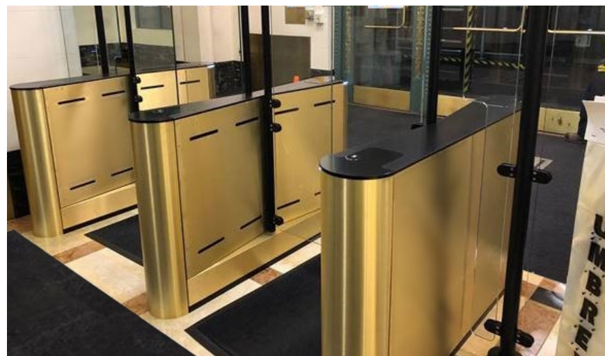
Fastlane Glassgate 200 turnstiles were installed to secure the entrance of the historic PG&E building.
